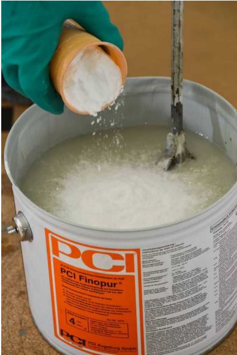
Peter Schuck's team added micro glass beads to the two components of the sealant. They ensure a non-slip surface.
