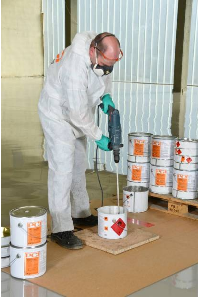
During the final step of the renovation work, the floor of the Paidi warehouse was sealed. For this purpose, the processors used the 2K PUR sealing PCI Finopur.
