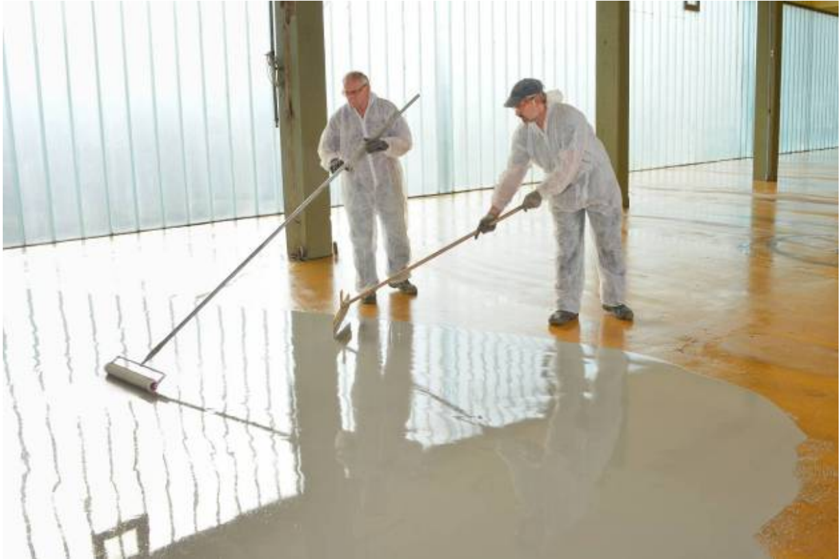
... a self-levelling floor coating that was spread over the entire area by means of notched trowels.
