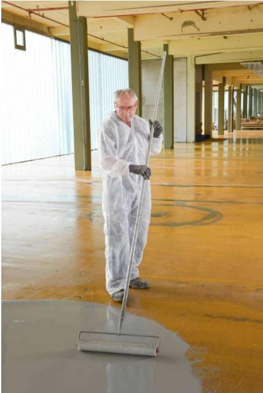
To level and vent the coating, the construction pros treated the applied product with a spiked roller.
