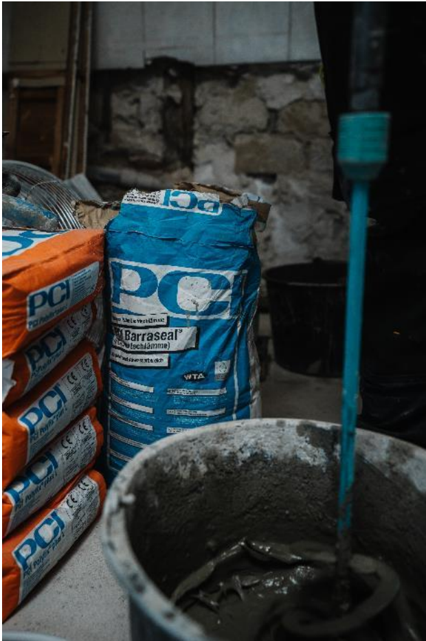
The craftsmen waterproofed the floor-wall transition with PCI Barraseal. ( Link to high-resolution photo)
