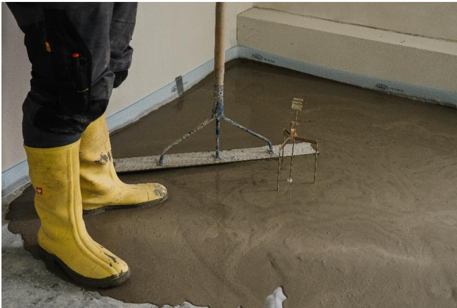
The flowable ready-mix mortar PCI Novoment Flow can be conveniently applied standing up. ( Link to high-resolution photo)
