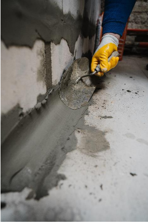
Interior waterproofing with PCI Polyfix Plus L to form a tight covering ( Link to high-resolution photo)
