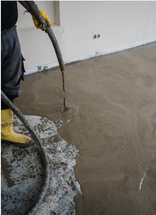
The screed PCI Novoment Flow is applied to the substrate waterproofed with PCI BT 21 without waiting time. ( Link to high-resolution photo)
