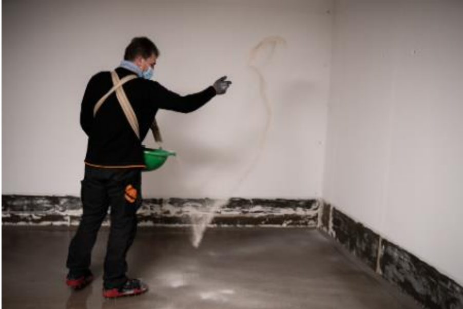
After application, the craftsmen sanded the fresh scratch coat PCI Apoten OS P in excess with quartz sand 0.3 - 0.8. (Link to the high-resolution Photo )
