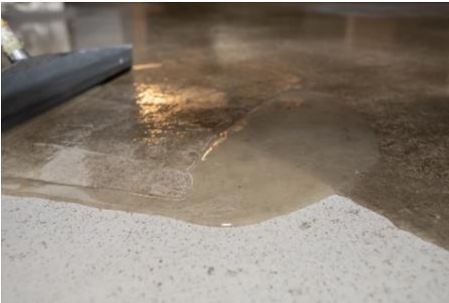
For the coating of the approximately 800 m 2 underground car park, the substrate was first primed with PCI Apoten OS P. (Link to the high-resolution Photo )
