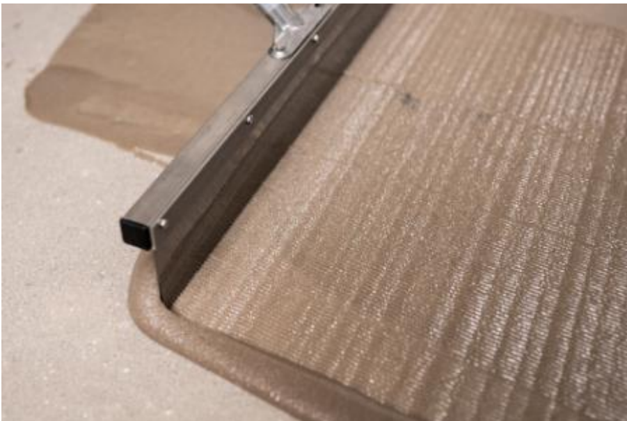
The scratch coat (PCI Apoten OS P with quartz sand 0.1 - 0.4) was applied to the primer applied the day before using a toothed squeegee. (Link to the high-resolution Photo )
