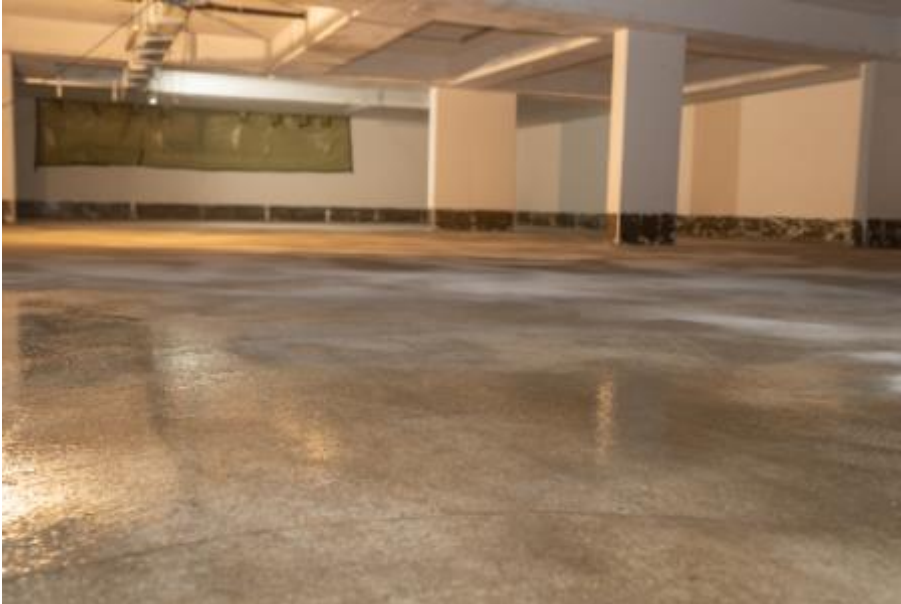
Completely primed with PCI Apoten OS P - the underground car park with 27 parking spaces under a newly built residential complex in Frechen. (Link to the high-resolution Photo )
