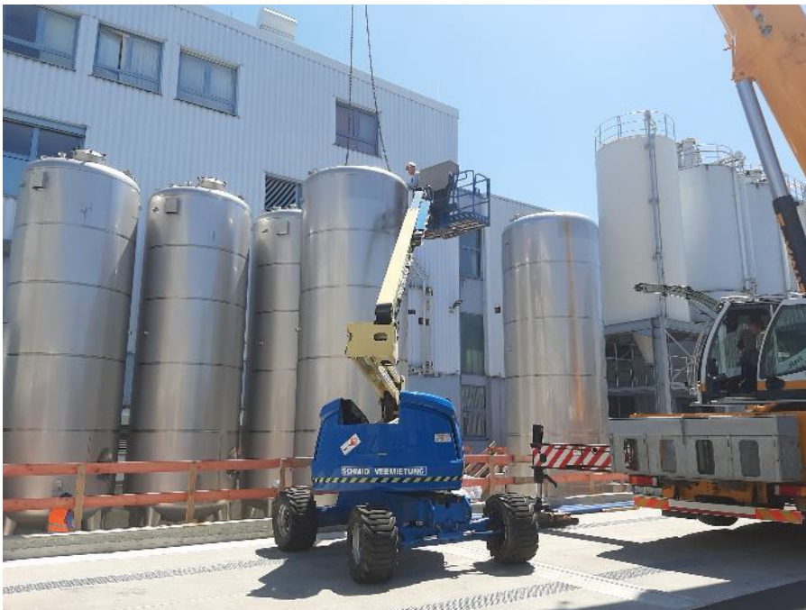
Part of the new dispersion plant will include seven additional raw material stainless steel tanks (construction phase in summer 2022). ( Link to high-resolution photo)
